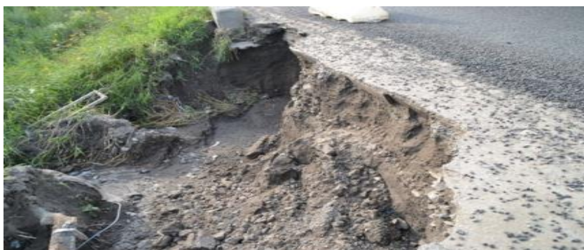
Figure 3. Destruction of the road in Hanoi
